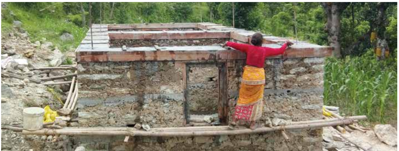
Home owner curing a concrete lintel band to make it more resilient after SDC technical support. Immediate Technical Support to Homeowners in Ramechhap (ITSHO) Project
