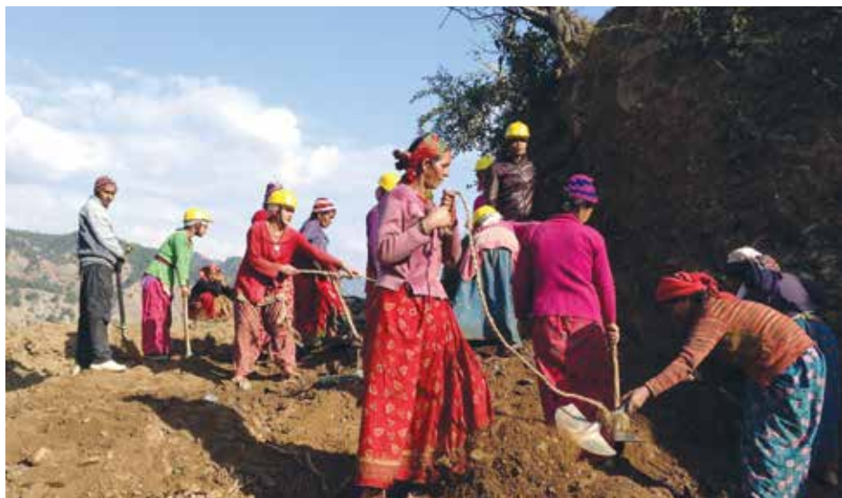
Members of local road users' groups engaged in the construction of Shreebhabar-Haat road in Baitadi. Aman Jonchhe
