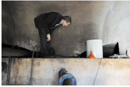
A Swiss expert inspecting the drinking water reservoir built in 1960 in the Croatian municipality of Fužine. © SECO
